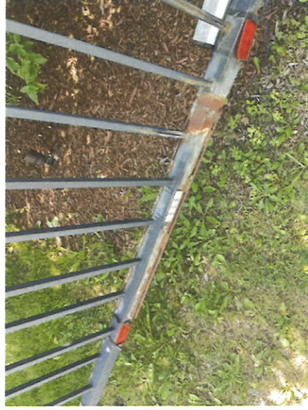
Gate rust (south entrance shown)
