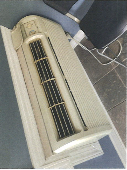
HVAC unit at south gate house
