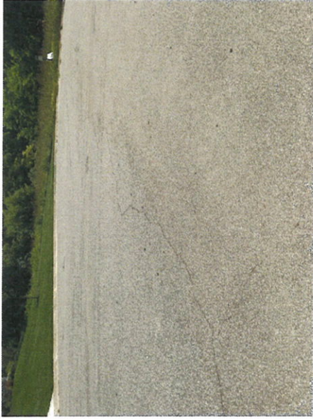
Phase 3 pavement cracks (Cambe Court shown)
