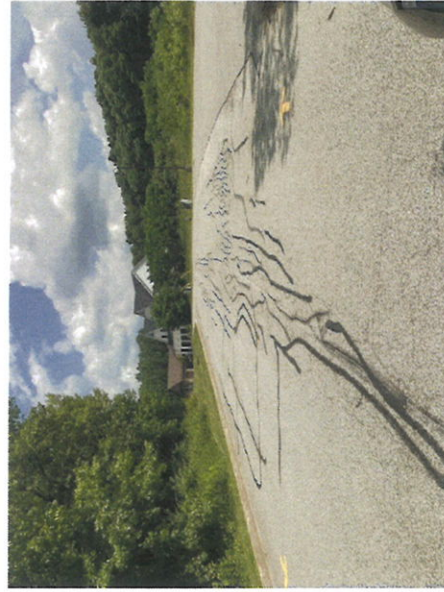
Phase 2 pavement cracks (Ketill Trace shown)
