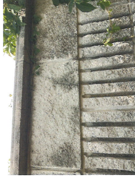
Masonry wall cracks
