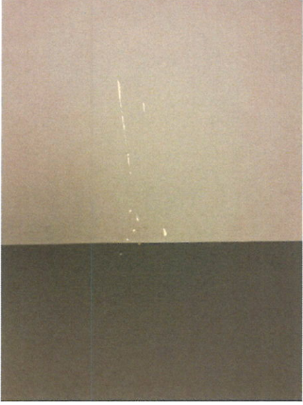
Paint finish deterioration
